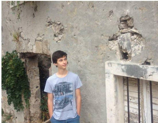
Bomb damage to house in Sućuraj.
